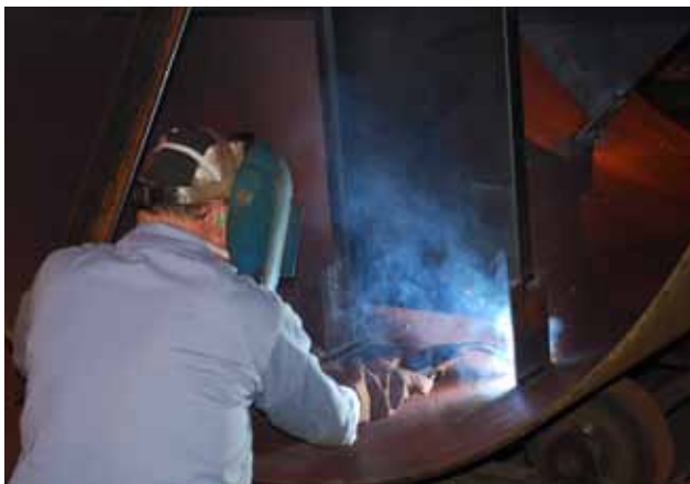
Baffles, relief valve flanges, and other openings are welded in place once the shell is complete.
