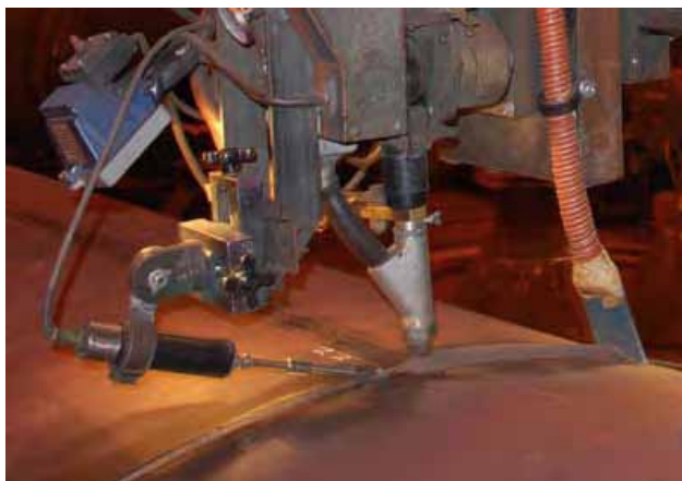
Submerged arc welding (SAW) is a process where the weld is performed under a shielded blanket of granular flux.
