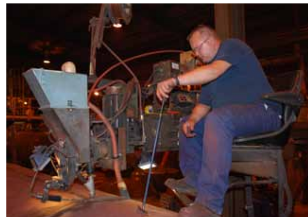
ASME code certified welders control and monitor the procedure from the pilot seat.
